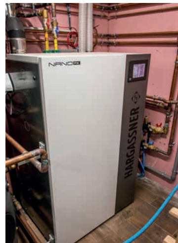
Chaudière Hargassner, 12 kW
