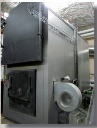
Chaudière Fröling LambdaMAT, 420 kW
